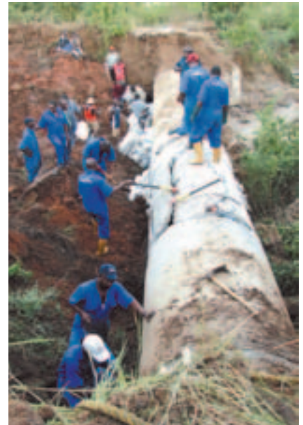
Indian and Chinese contractors are playing an important part in the country's water provision facilities
